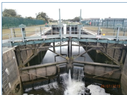
Photograph showing the upstream and middle lock gates. The paddles in the middle (ebb) gates are permanently cracked open to maintain a flow of water through the lock. This helps to disperse silt laden water drawn down from the upstream reach.
